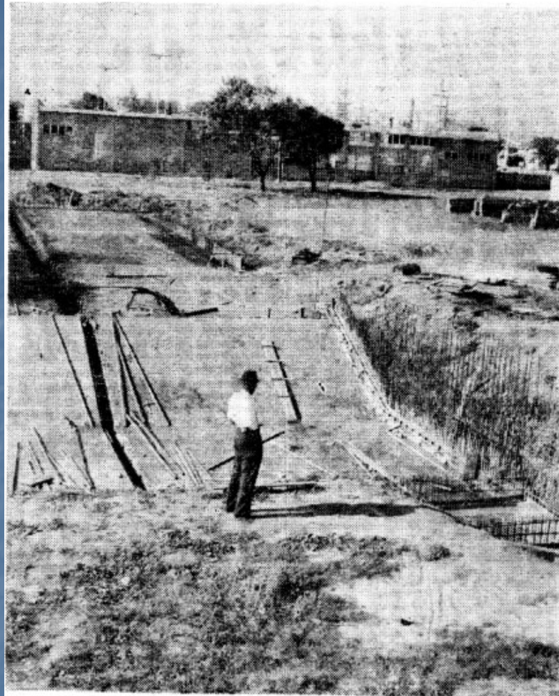
Excavations and foundation works on the BHP's "gift" swimming pool in Dangar Park, Mayfield East, are nearing completion. Picture shows progress on the $160,000 (£80,000) project.
